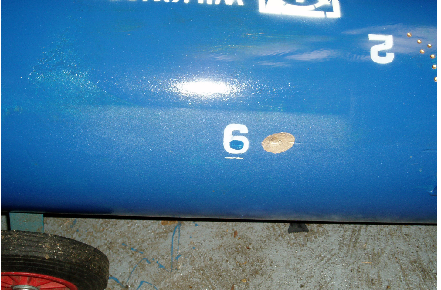
PHOTO 6: LOCAL WALL THINNING
