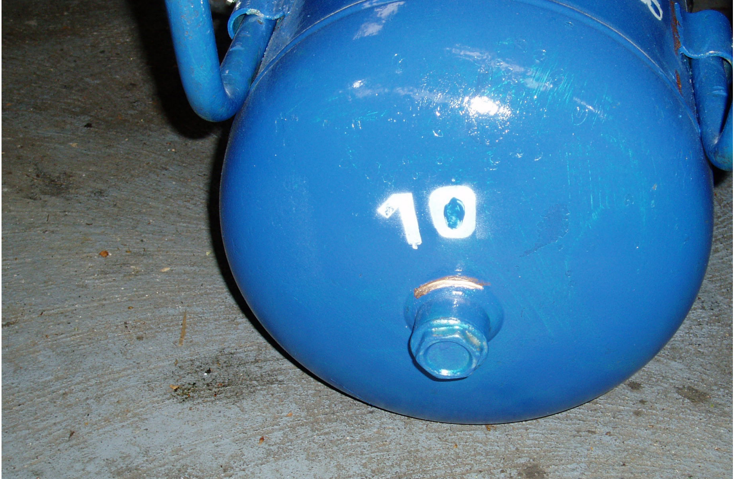
PHOTO 10: NOZZLE N4 WELD GRIND DEFECT
