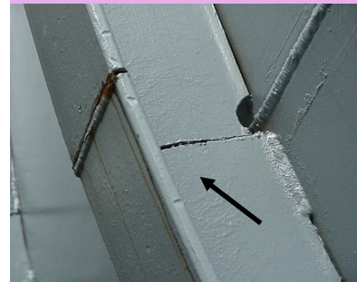
Failed stiffener weld
