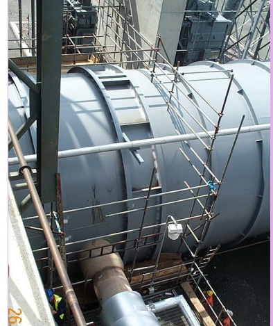
The steam duct
