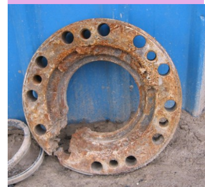
The failed flange
