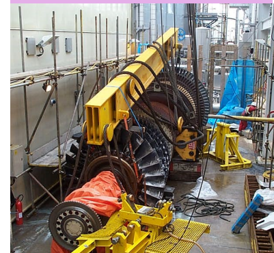
The dropped turbine rotor
