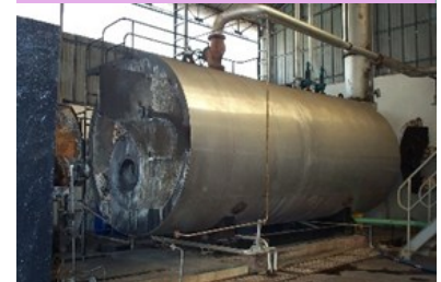
Boiler door blown off
